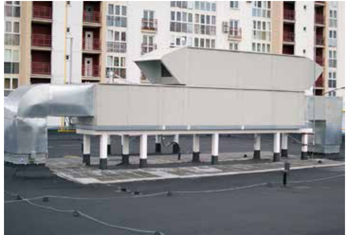
Figure 3: Air Handling Unit in metal box enclosure on rooftop of commercial building.
