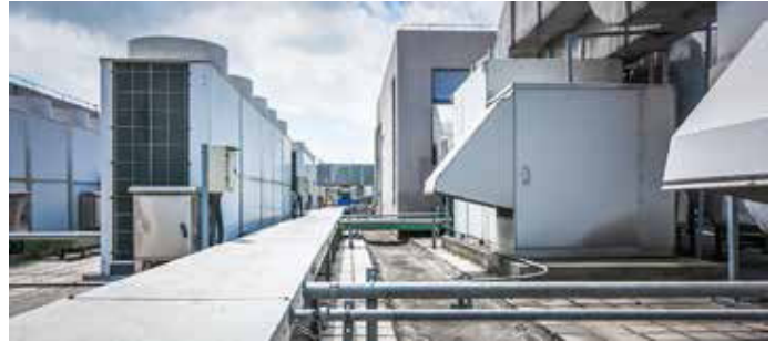
Figure 1: Square air-conditioning unit on a roof with a fan
